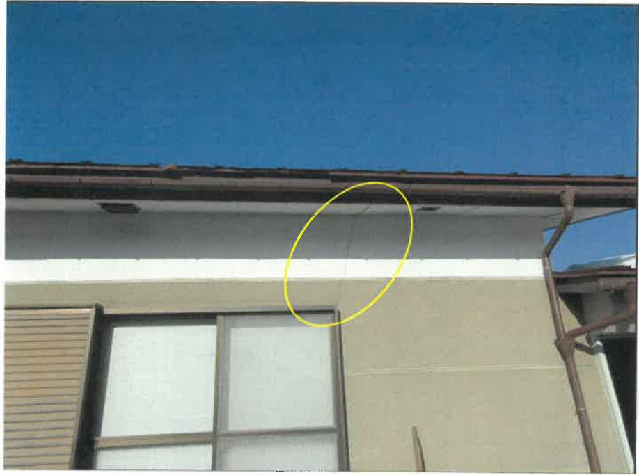
物件2:外壁の亀裂
